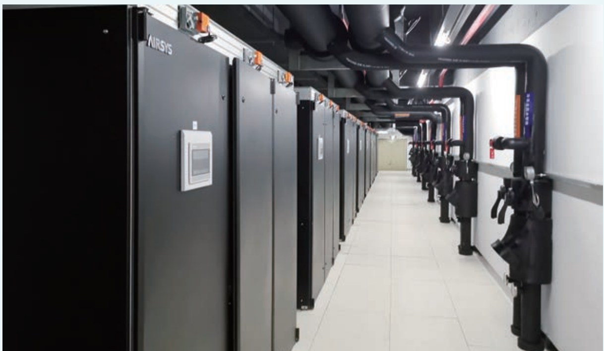
Existing IDC Equipment Sale and Leaseback Project of SZZT Electronics
